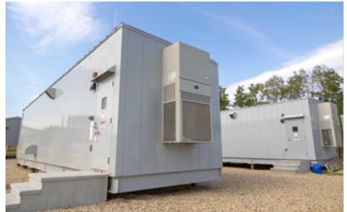
Figure 7: The Energy Distribution and Battery Storage Systems at E.L. Smith.
